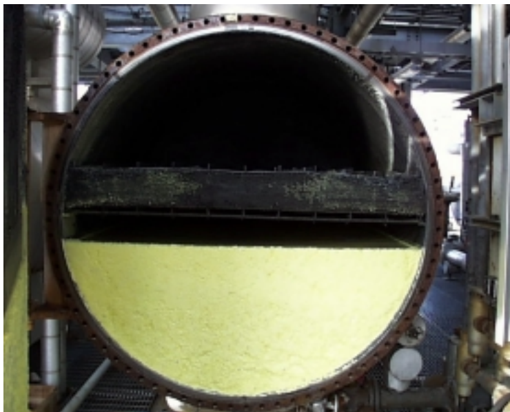
Figure 5.3.12B: Sulfur in No. 4 Sulfur Condenser as a Result of a Plugged Seal Leg
