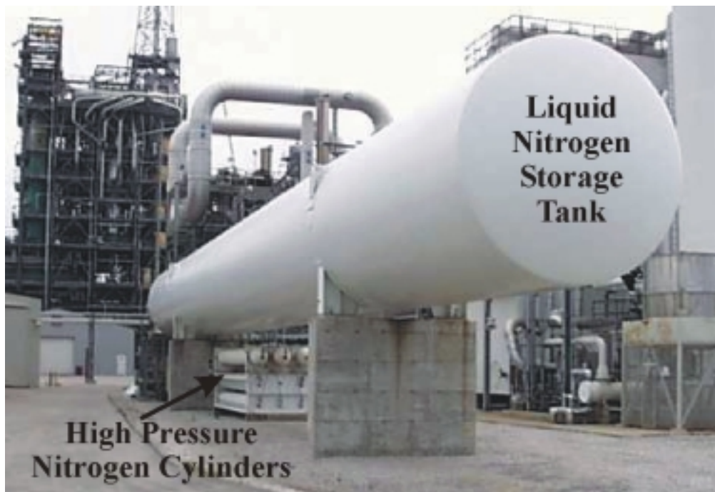
Figure 5.1.7C: Liquid Nitrogen Storage Tank and High-pressure Cylinders
