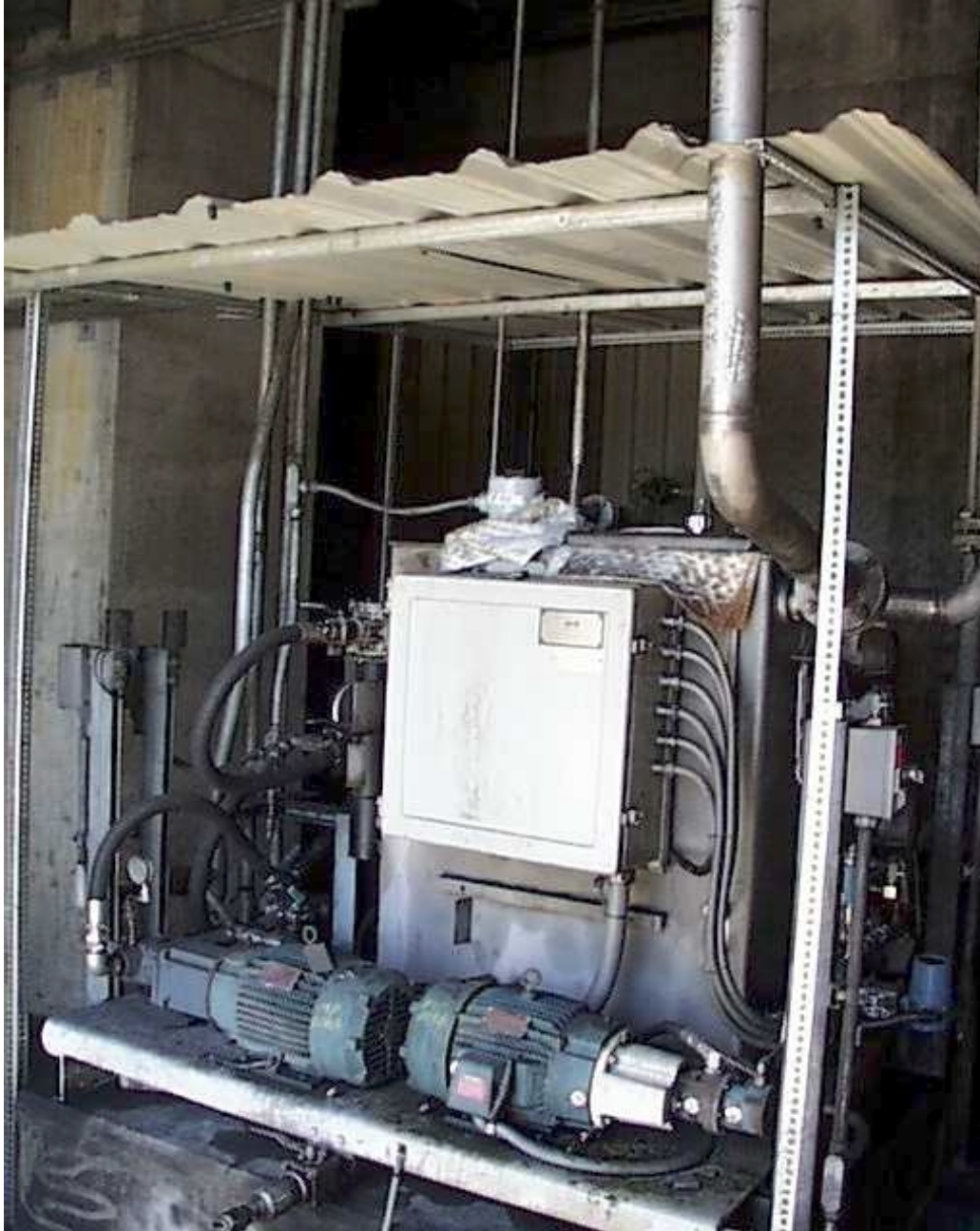
Figure 5.2.2C: Rod Mill Lube Oil Skid
