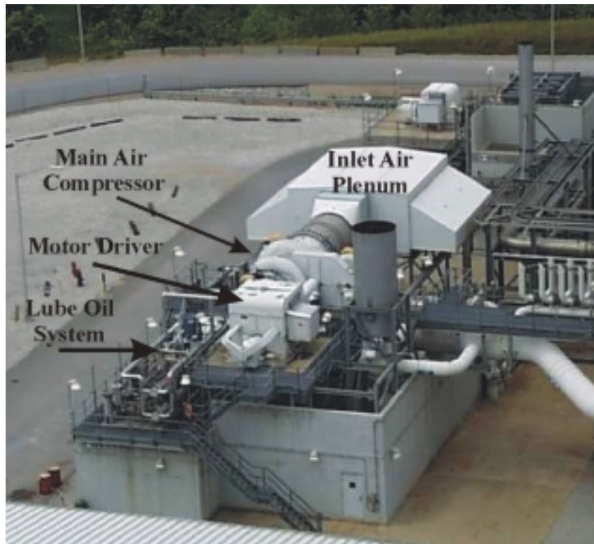
Figure 5.1.1A: Main Air Compressor
