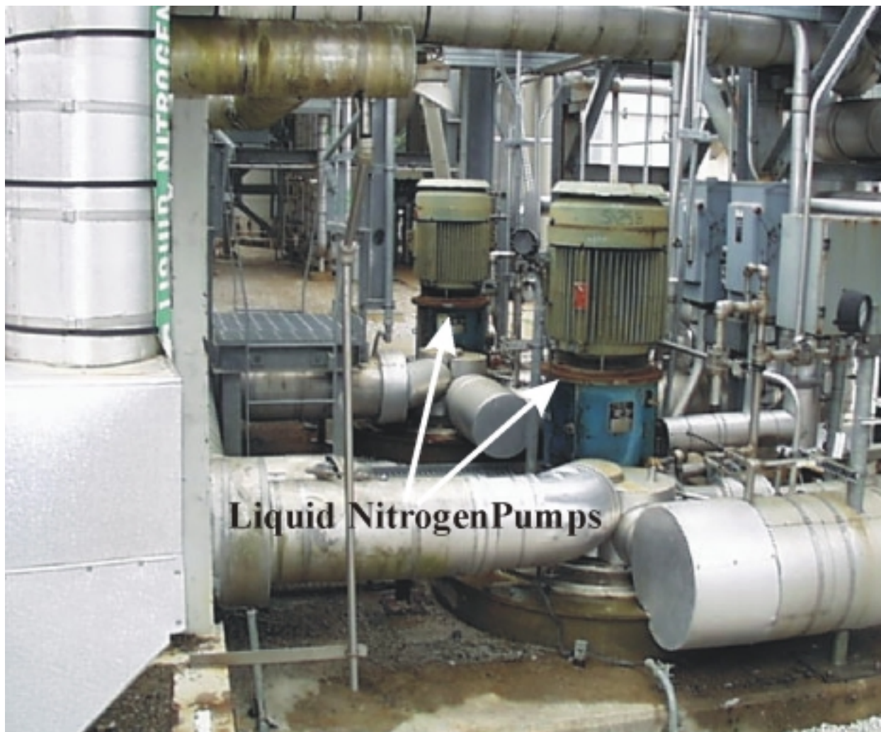
Figure 5.1.7A: Liquid Nitrogen Pumps
