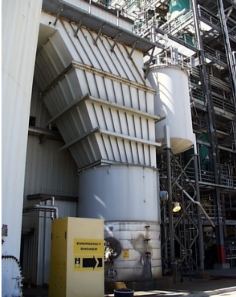
Figure 5.3.4B: Slag Fines Settler
