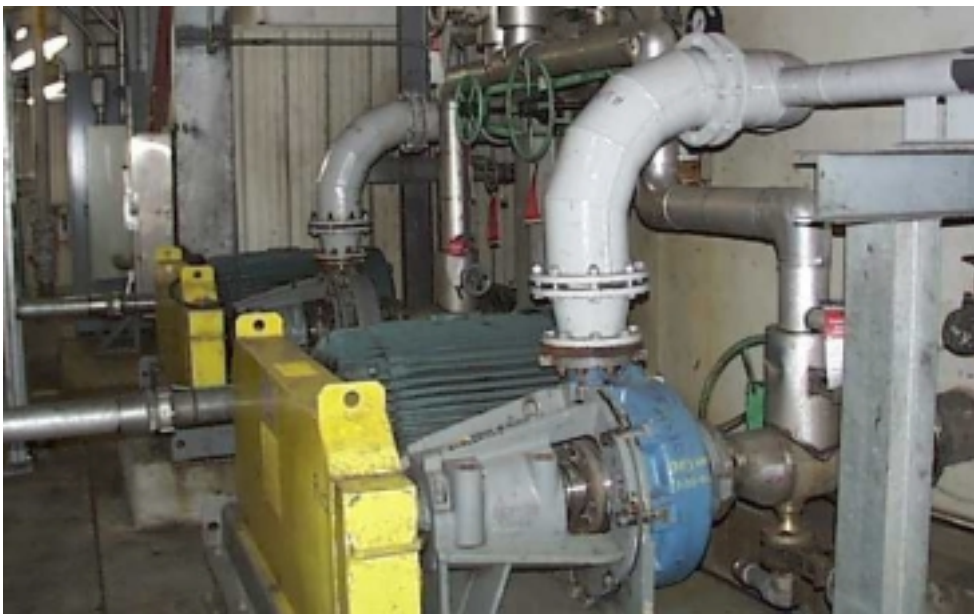
Figure 5.2.3B: Slurry Recirculation Pumps
