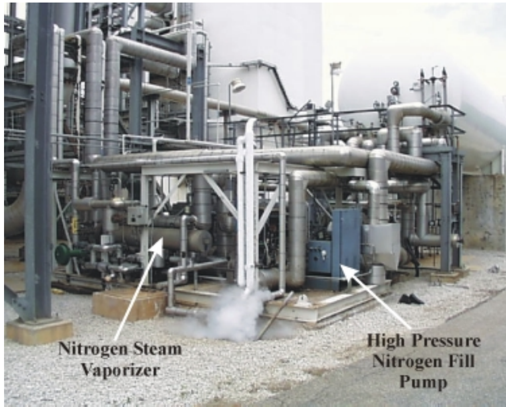
Figure 5.1.7B: Liquid Nitrogen Pump Skid
