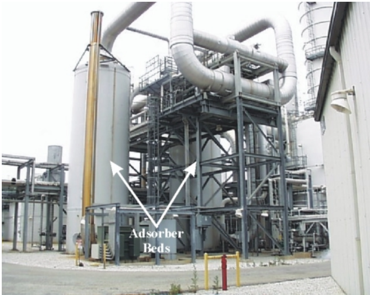
Figure 5.1.3A: Adsorber Beds for the Air Purification System
