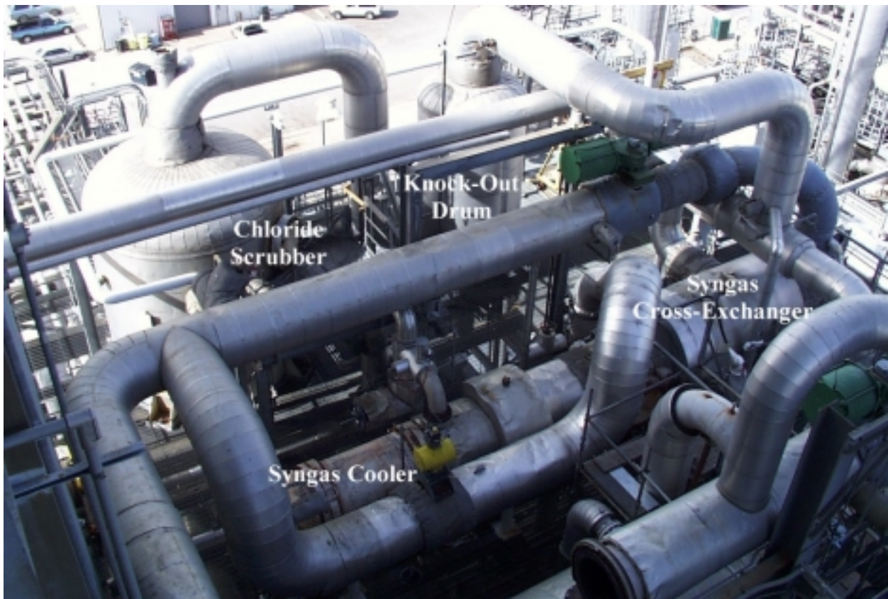
Figure 5.3.7A: Major Equipment Associated with the Chloride Scrubbing System
