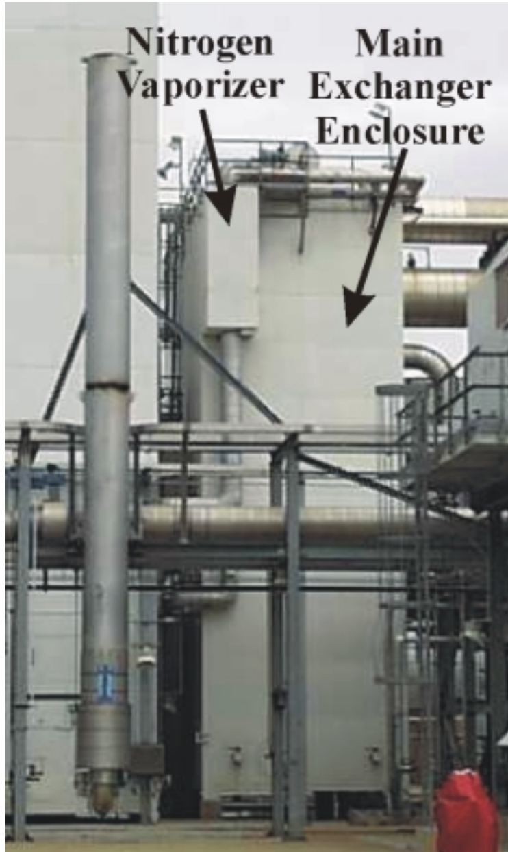
Figure 5.1.4A: Nitrogen Vaporizer and Enclosure for Main Exchangers
