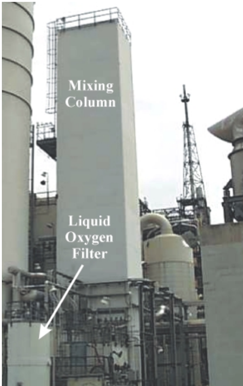
Figure 5.1.6A: Equipment Associated with Oxygen Mixing System
