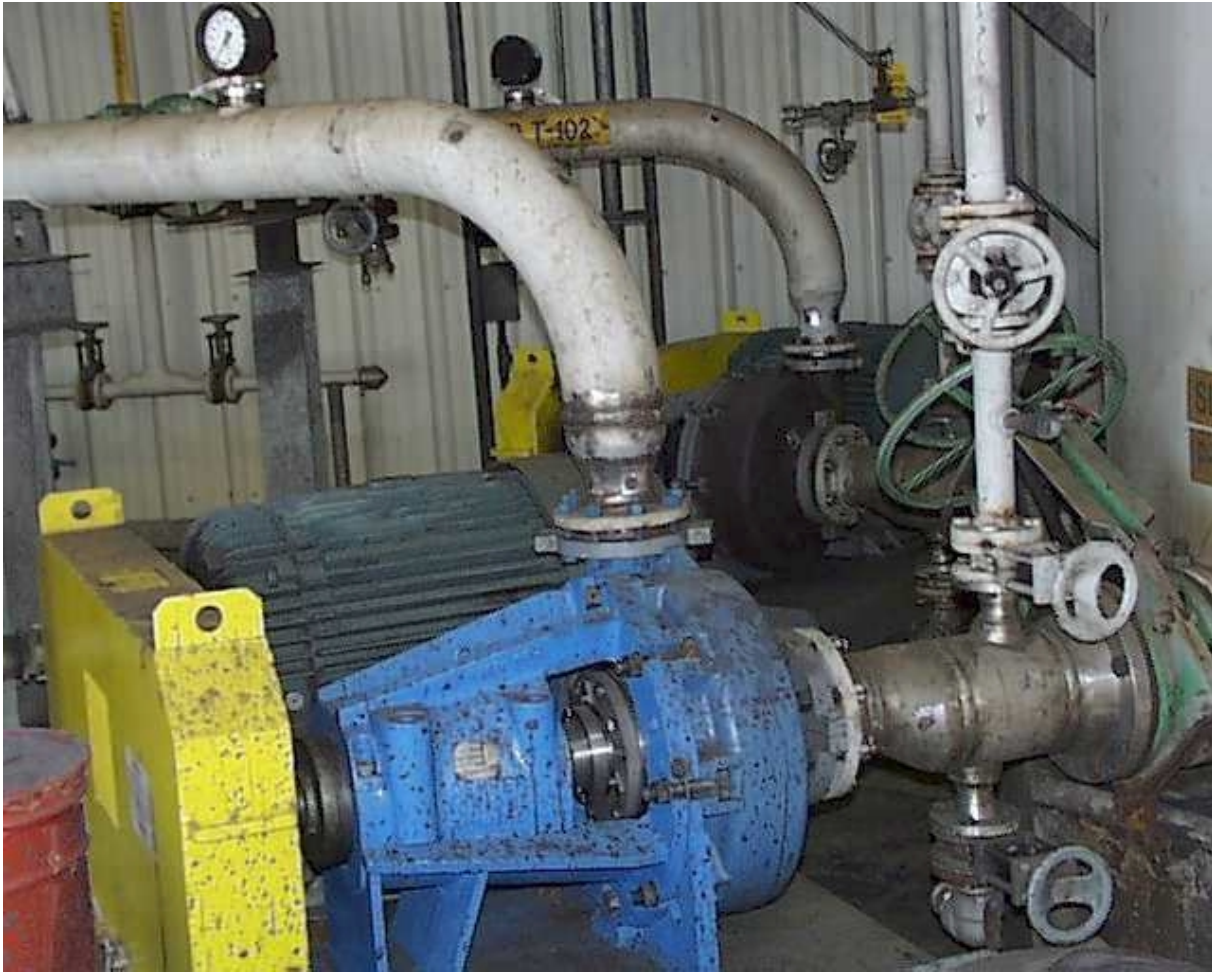
Figure 5.2.2B: Rod Mill Product Tank Pumps
