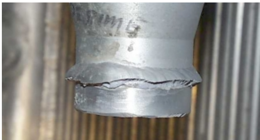
Figure 5.1.4D: Derime Header Failed Weld
