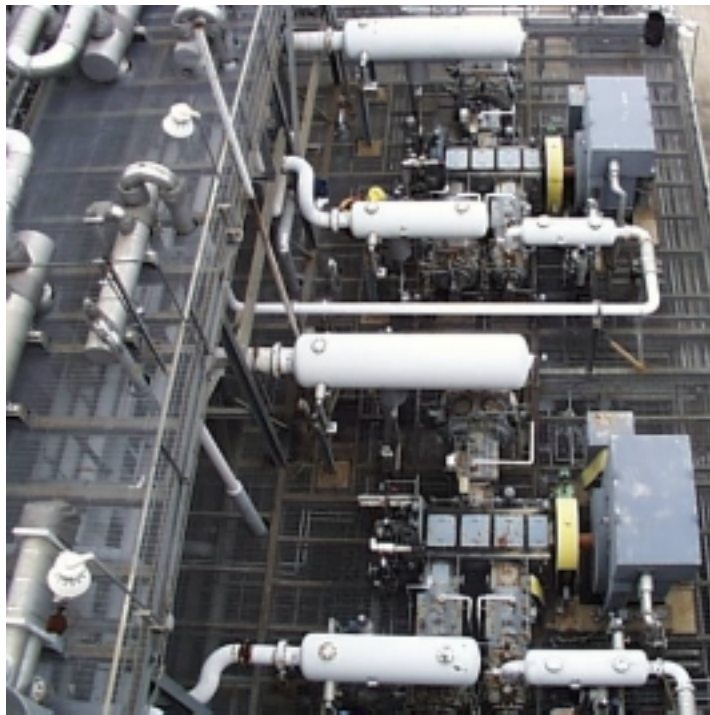
Figure 5.3.12C: Tail Gas Recycle Compressors
