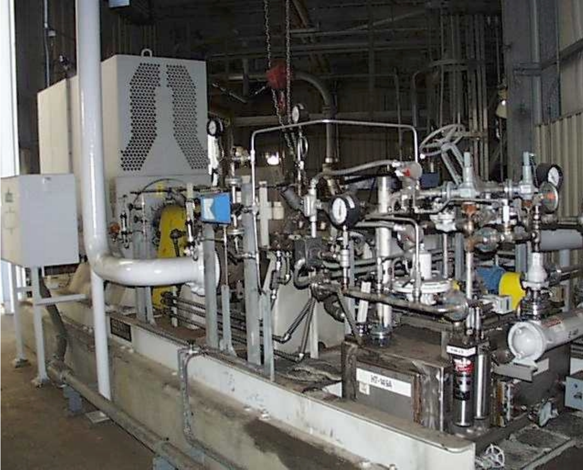
Figure 5.3.4D: Slag Quench Feedwater Pumps
